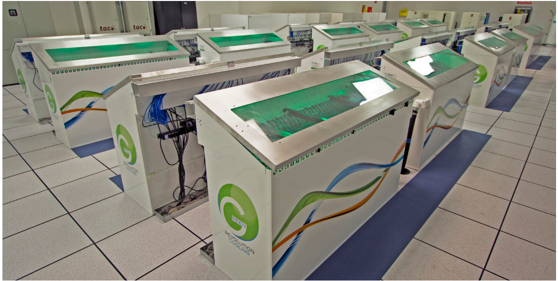
Submersion-cooled racks installed at CGG in Houston, Texas
